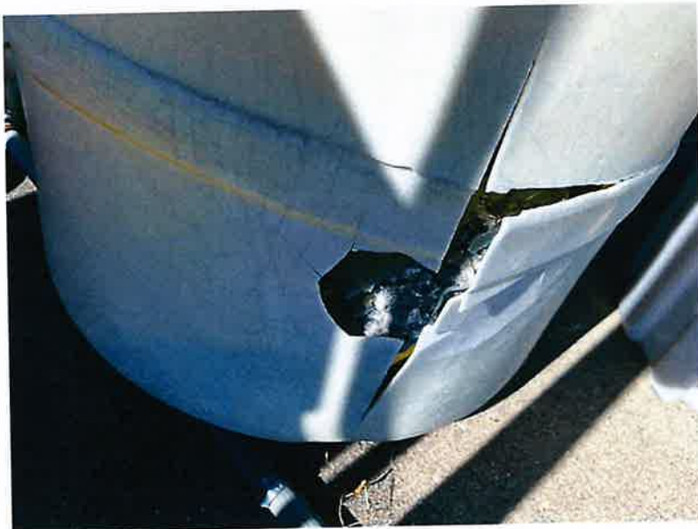
Fuel Island. Yellow barrel absorbent material damaged.
